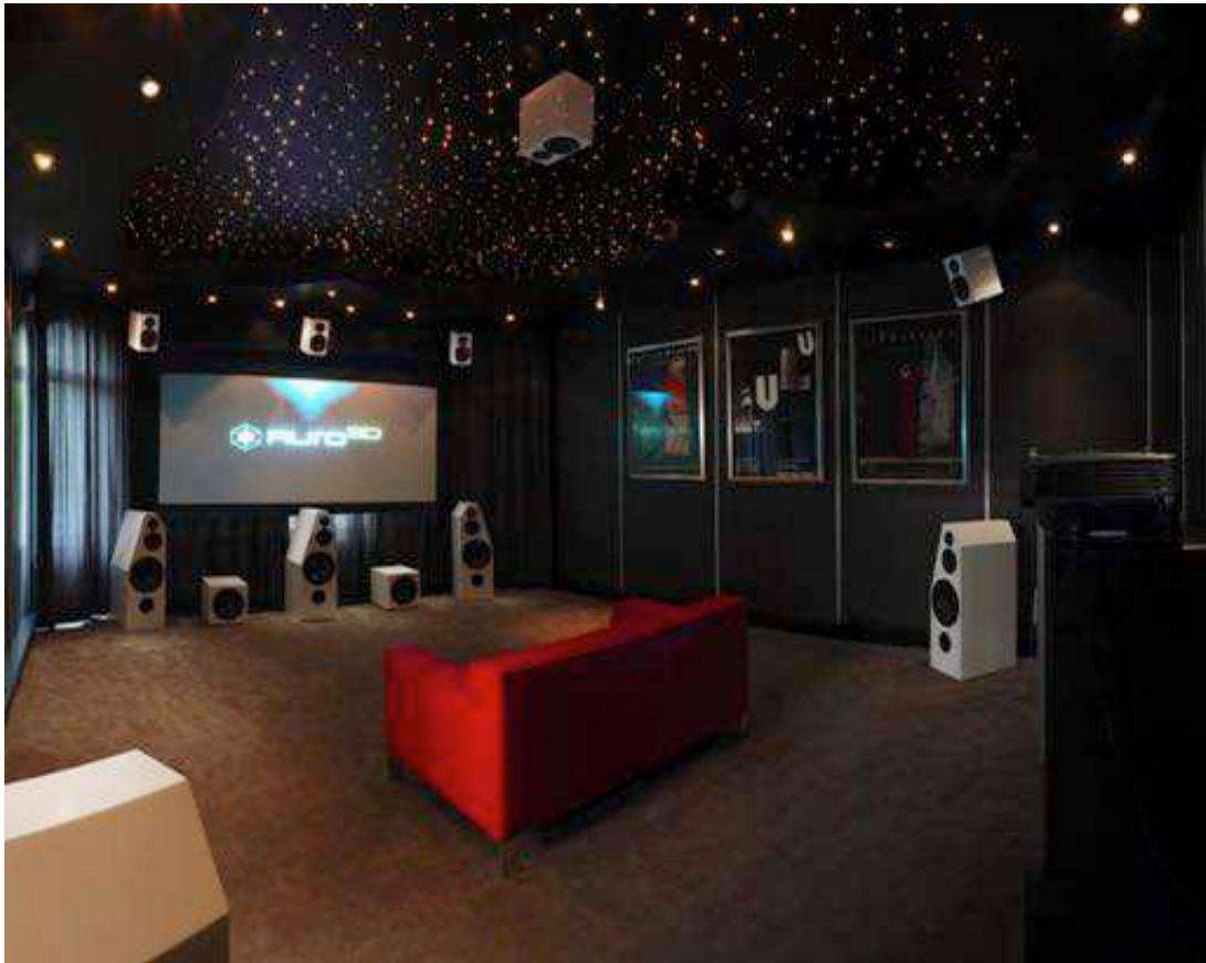
Auro 11.1 Certified Home Cinema install at demo room of Stassen Hifi (The Netherlands).
